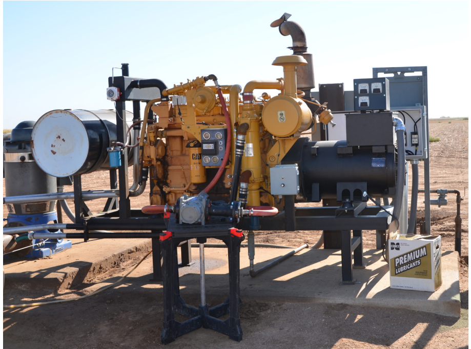
Natural gas Caterpillar 3306TA driving a Marelli three-phase generator, providing power to three irrigation wells.
